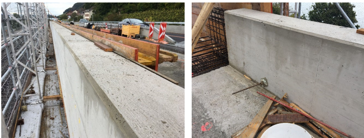
Figure 5 – Appearance of the concrete surface after demoulding.
